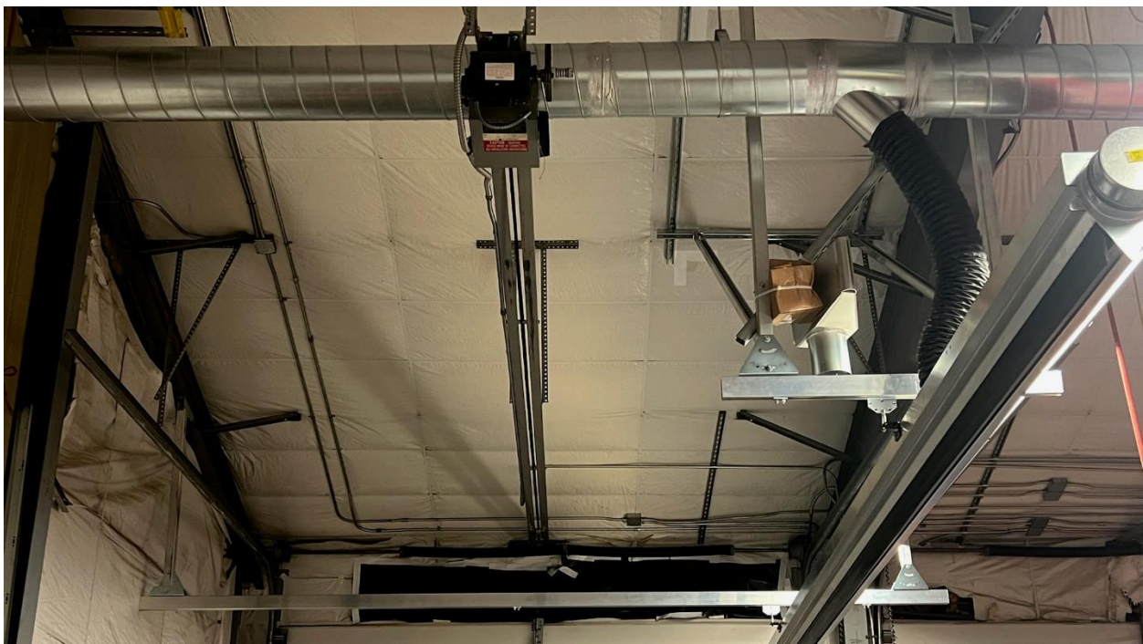
Figure 32. Inoperative Overhead Door Motor, Bay 4
