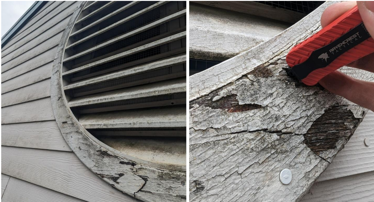
Figure 30. Station 93 Exterior Trim Dry Rot
