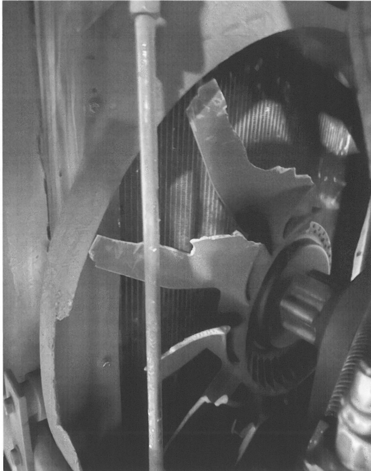
Figure 3. Engine 94 Fan, Shroud, and Radiator
